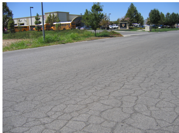
Figure 15: The severely cracked condition of Santa Anita is not what was expected.
