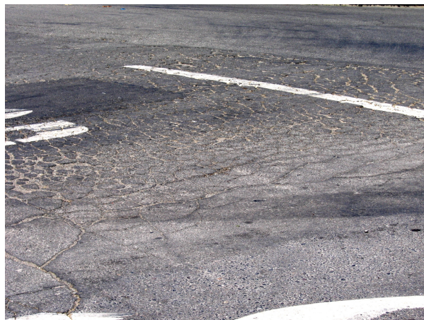
Figure 13: Harter Avenue control section condition in 2007.
